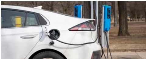
ON-STREET EV CHARGING
