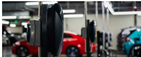
OFF-STREET EV CHARGER INSTALLATIONS
